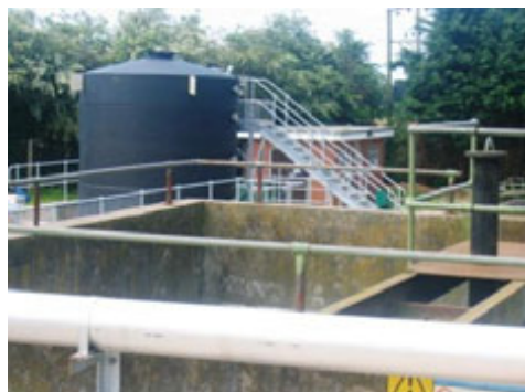
Fownhope Waste Water Treatment Works Not the prettiest view but essential
